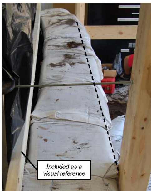
Figure 9. Permanent wall displacement as observed during wall deconstruction.
